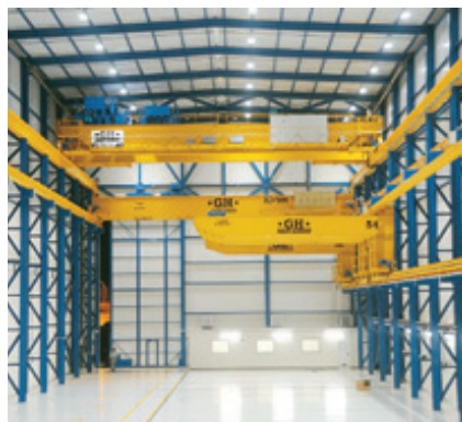
Double girder crane and cantilever crane
